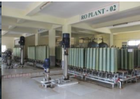
Reverse Osmosis Plant
