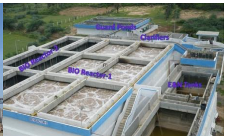
Effluent Treatment Plant
