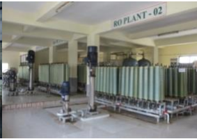
Reverse Osmosis Plant
